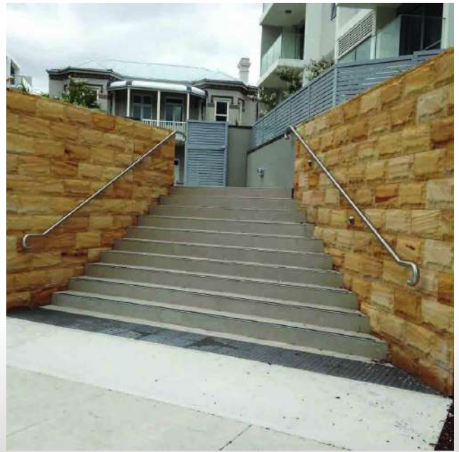
SANDBLASTED CHIPPED EDGES
